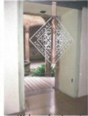
Wide and automatic door, smooth surface. This door can be difficult for visually impaired to use due to the invisible glass...
